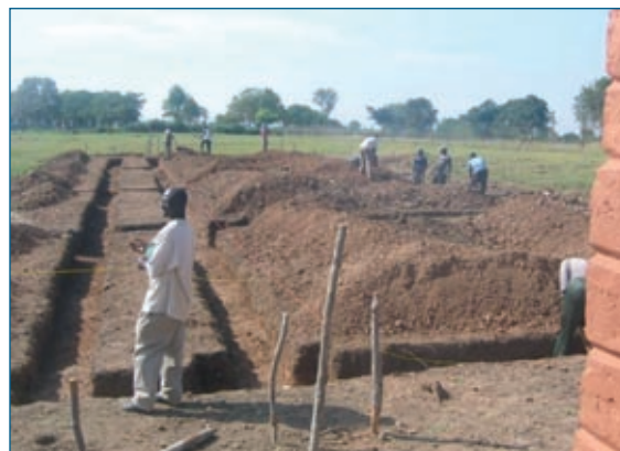
August 2007: Preparing to lay foundations for the second classroom block and library.
